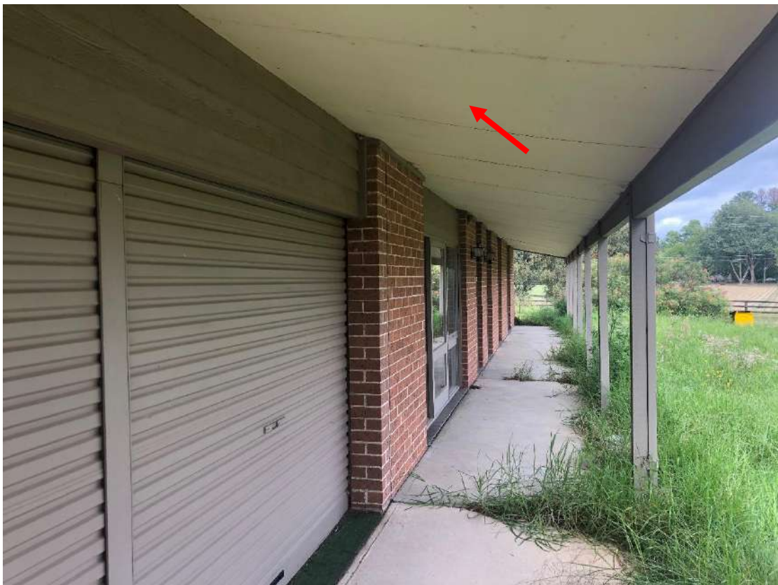
Photo 2: Existing dilapidated residential dwelling within southern portion of site looking north-east showing potential hazardous construction materials
