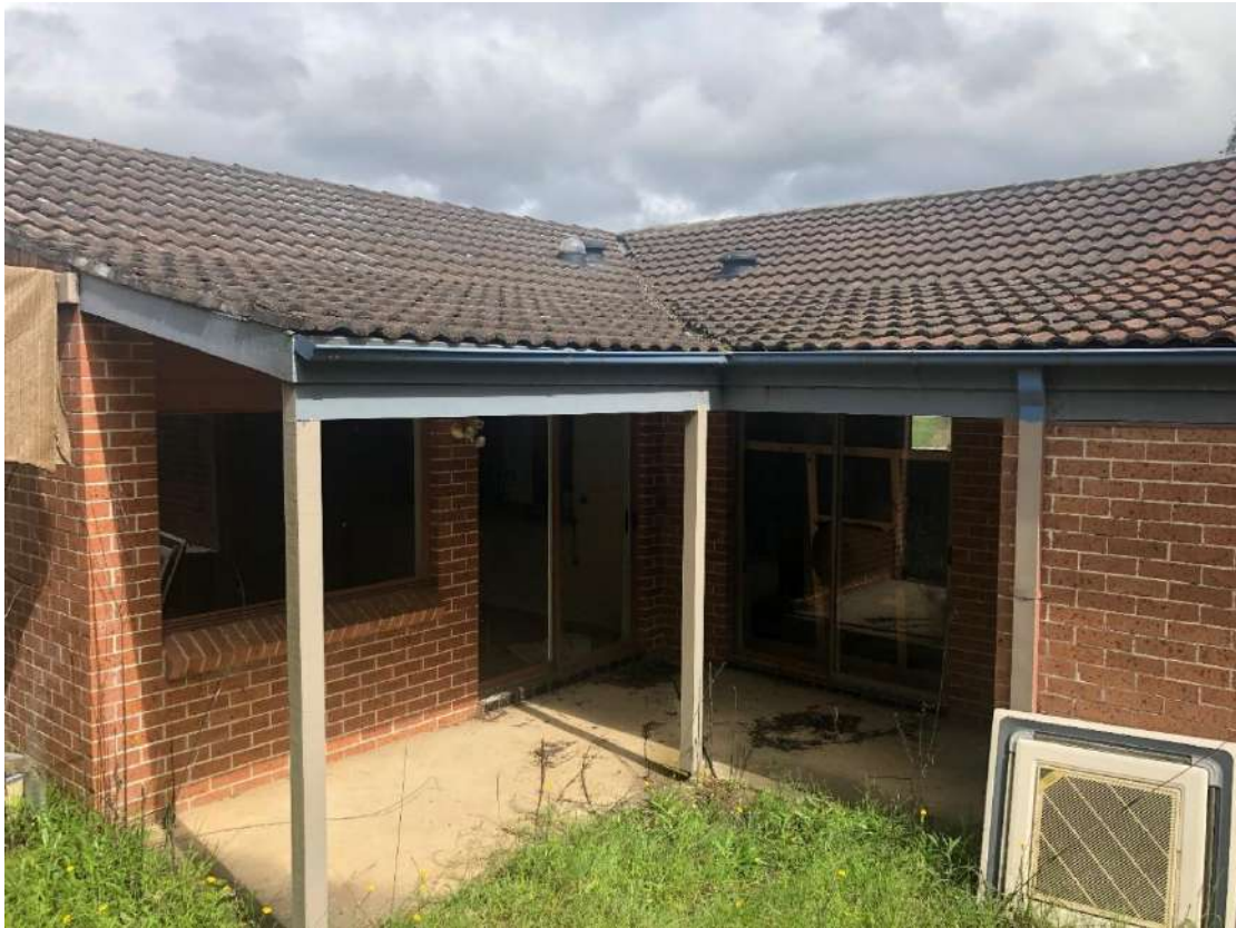
Photo 1: Existing dilapidated residential dwelling within southern portion of site looking north
