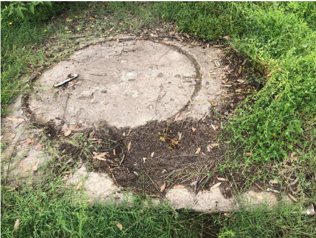
Photo 9: View of remnants of a concrete footprint area for a potential aboveground holding tank
