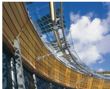
PV cells within glazed roof shading system
