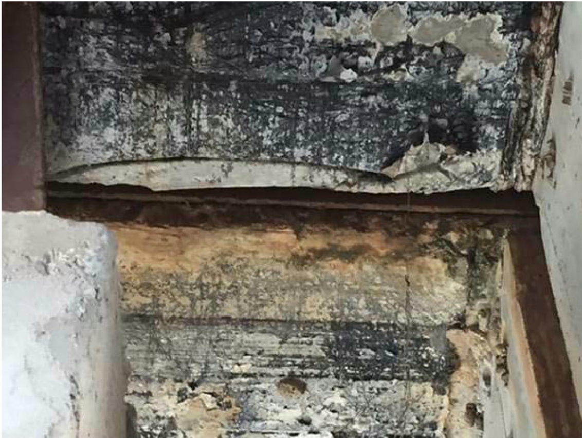
Photograph 4 Crevices between concrete formwork in Ropes Creek Bridge
