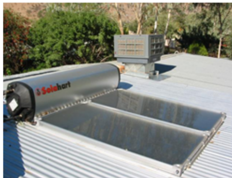
Figure 16 Solar hot water system
