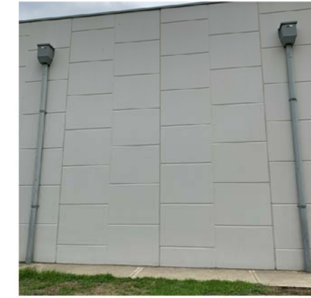
Existing pre-cast concrete panels to be retained. Existing downpipes to be retained.
