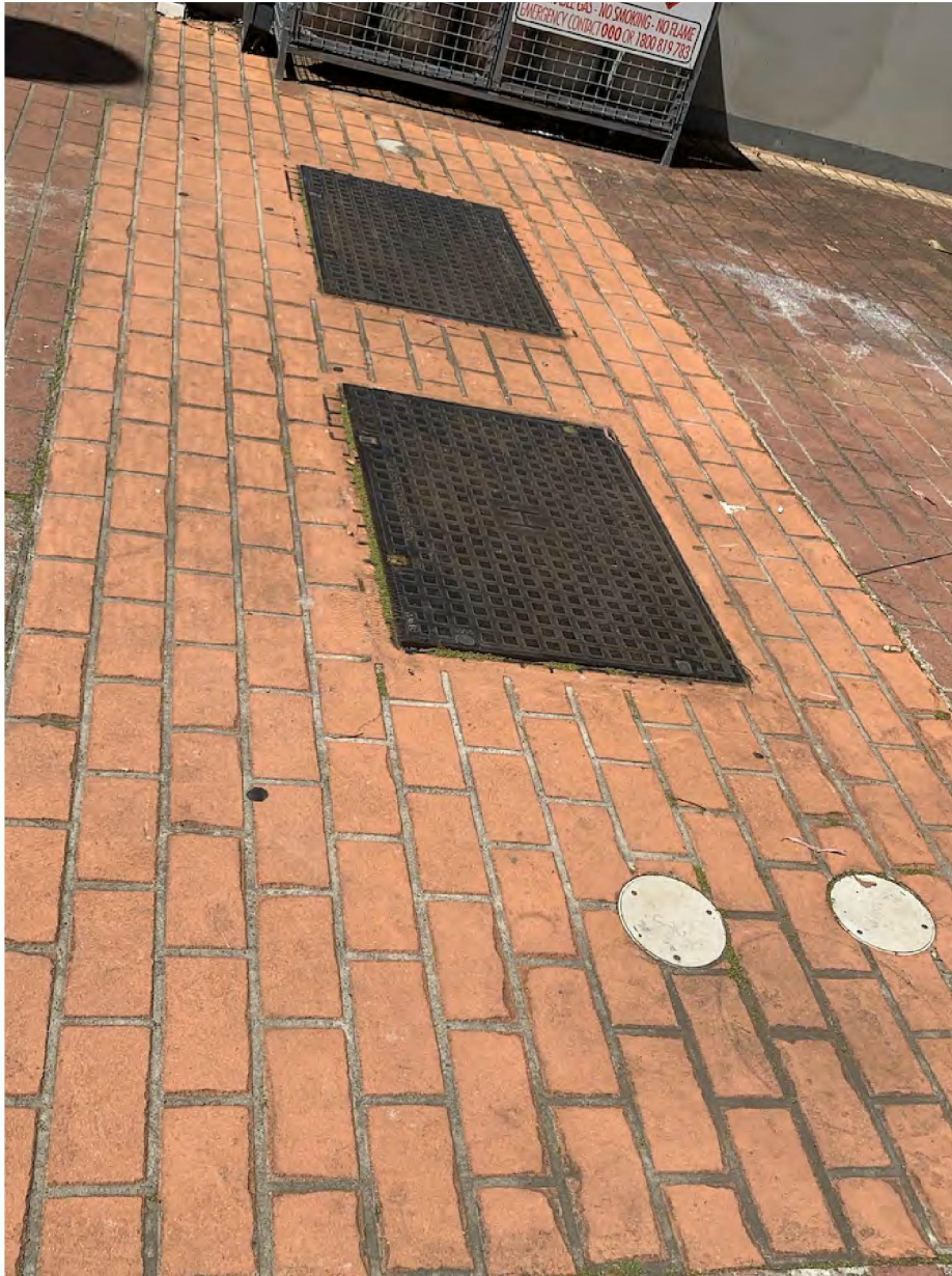
Photograph 9: There are three (3) grease traps serving the food outlets at the site.
