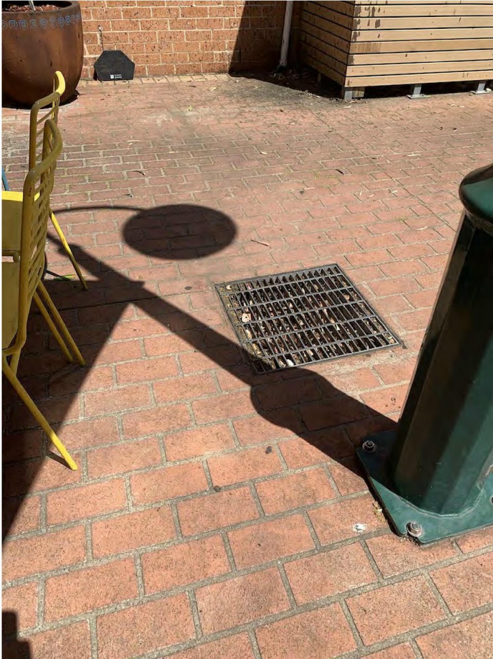
Photograph 7: Drainage is assisted by three (3) grated pits
