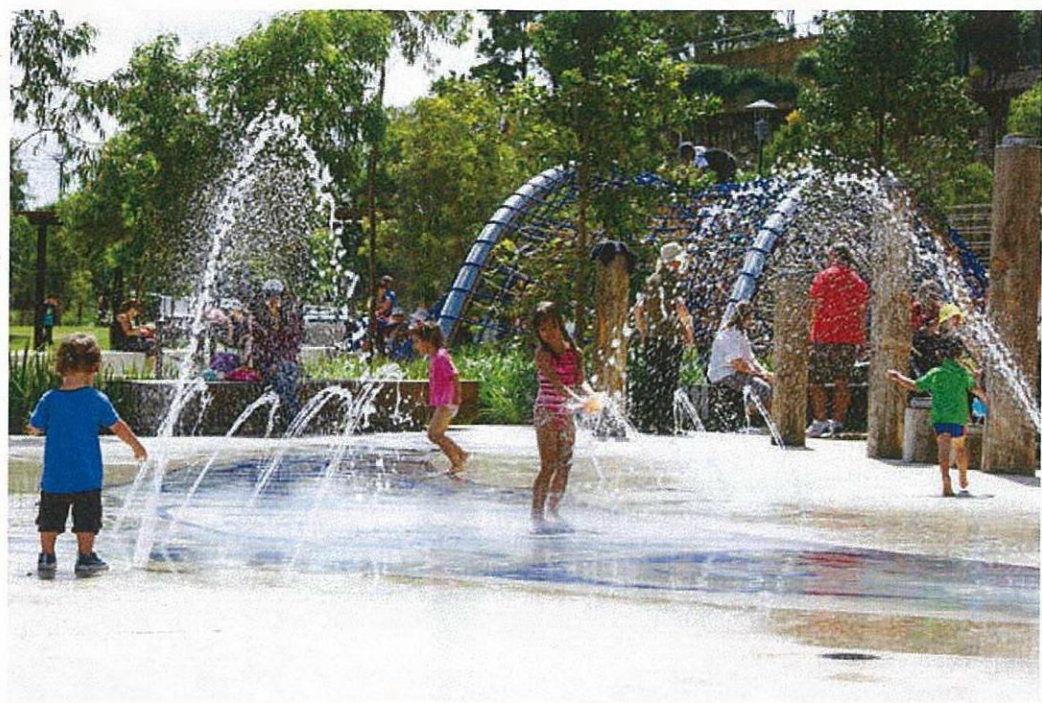
2 WATER PLAY WITH WATER JET COMING UP FROM GROUND
