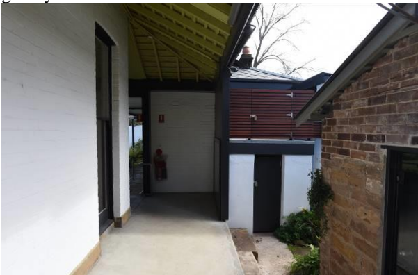
Figure 7: External southern façade of living room gallery, showing the former tank stand and location of bricked-in door.
