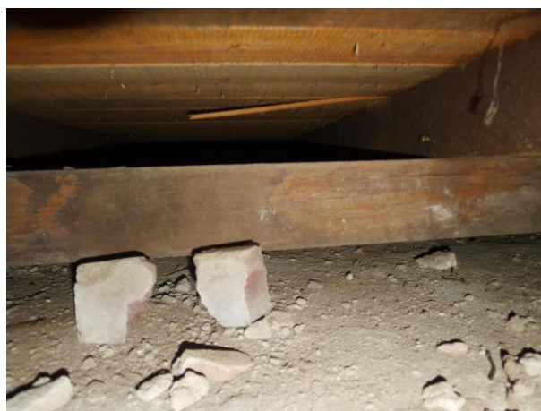
Figure 10: View of floor substructure of Living Room Gallery. Bearers are largely propped by bricks.
