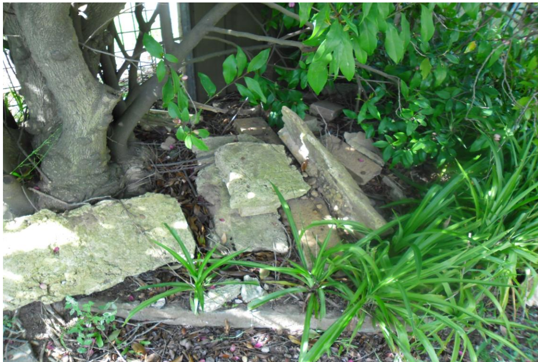
Photo 2 - Concrete Pieces Found in Front Yard of Number 28 (DP 2015)
