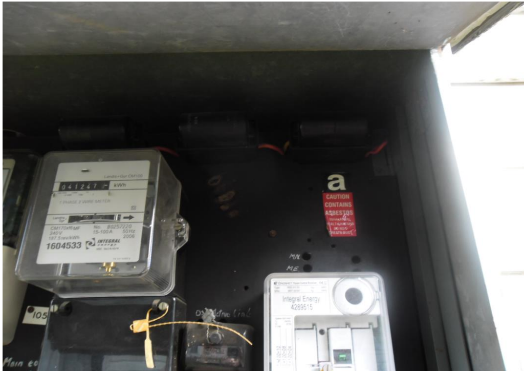
Photo 3 - Asebstos Warning in Electrical Box of Number 28 (DP 2015)
