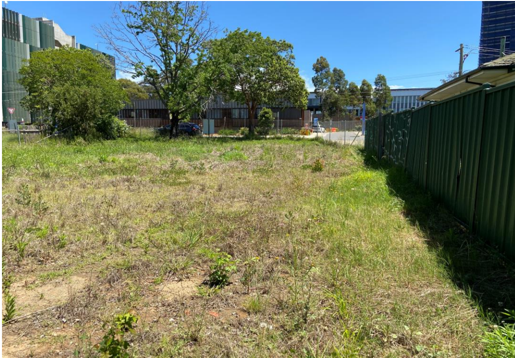
Photo 15 - Building/Demolition Waste (concrete and tiles) on Number 32, no significant change since 2015 (DP 2020)
