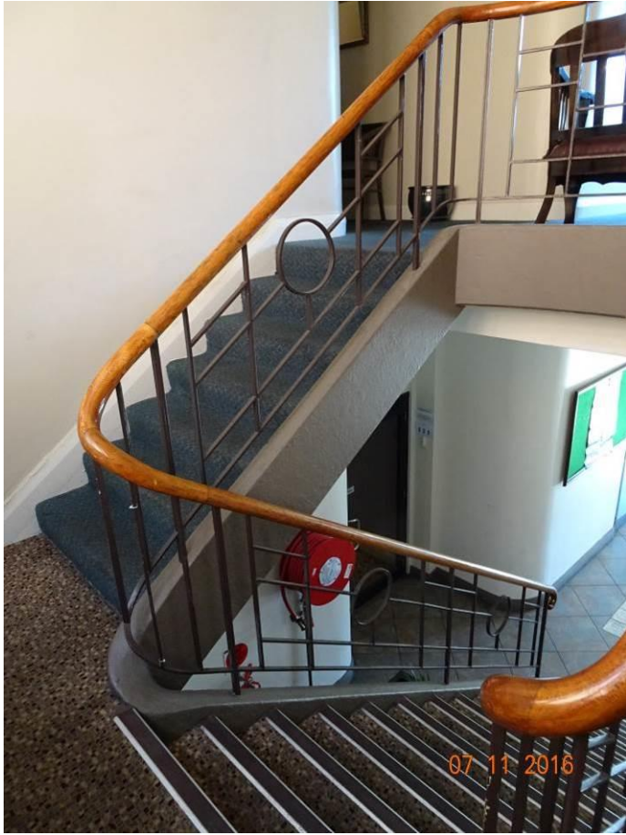
Figure 41: Stair balustrade and curved handrails
