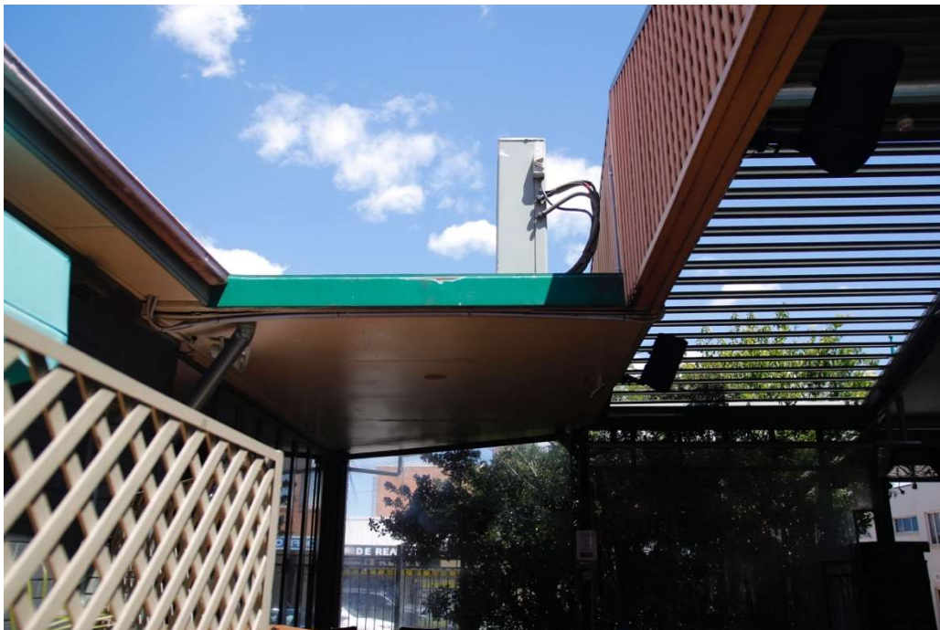
Figure 4: View of flat roof connecting Hotel to Beer Garden gable. Flat roof to be extended and air conditioning unit relocated to concealed position on new Gaming Room roof.
