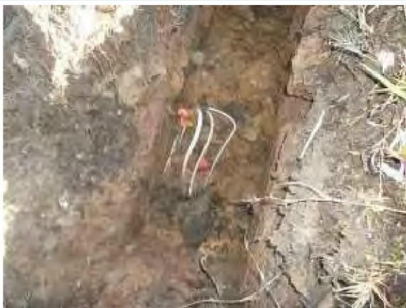
Photo 5. Underground service encountered at approximately 1.0 m BGL in TP12.
