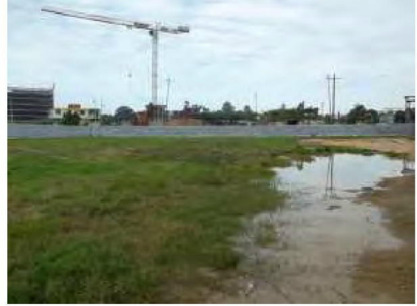
Photo 2. Water pooled on the surface of the site.
