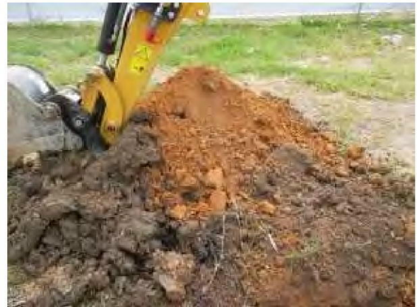
Photo 11. Fill and natural soils stockpiled adjacent test pit.
