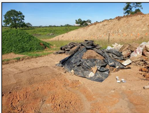
Photo 17: 19 March 2020: Stockpile of residual asbestos waste at time of classification. Stockpiled VENM in background.
