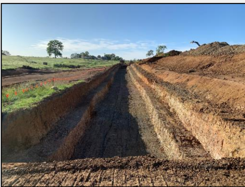
Photo 11: 28 February 2020: Overview of containment cell and exposed excavation faces. Waste placed in bottom of cell.
