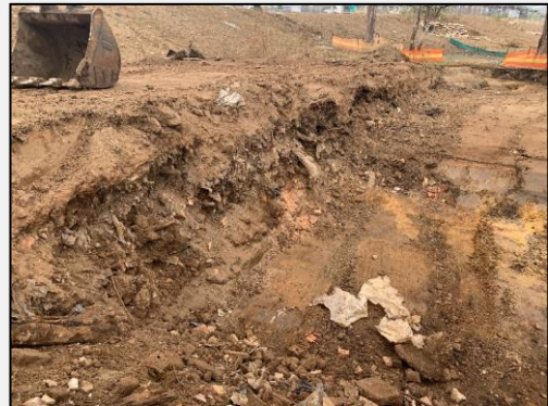
Photo 2: 08 January 2020: Commencement of excavation in remediation zone. Foreign materials including ACM observed.
