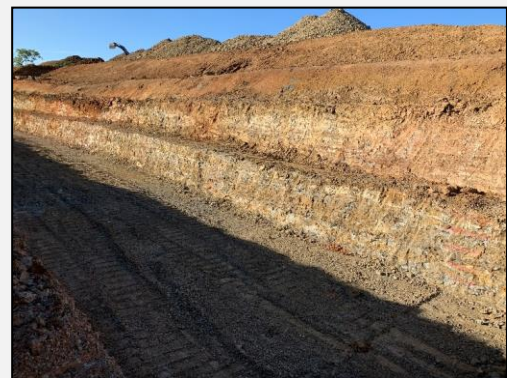
Photo 12: 28 February 2020: Overview of containment cell and exposed excavation faces. Waste placed in bottom of cell.
