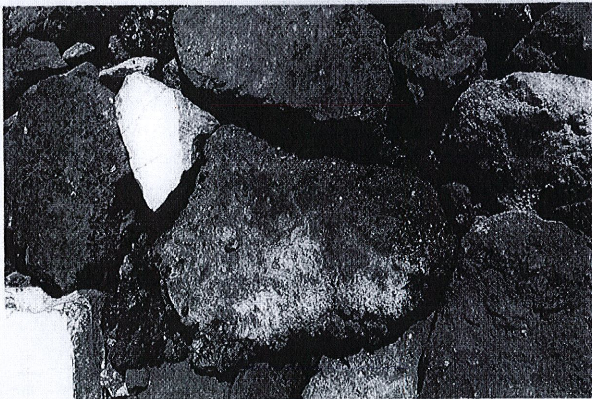
F: Stain 2 - Asphalt
