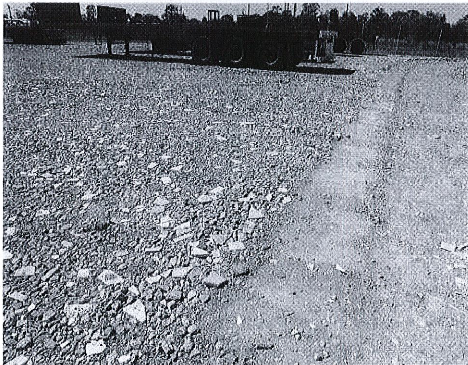
B: Recycled Crushed Concrete & Interface of Recycled Crushed Concrete and Underlying Material.
