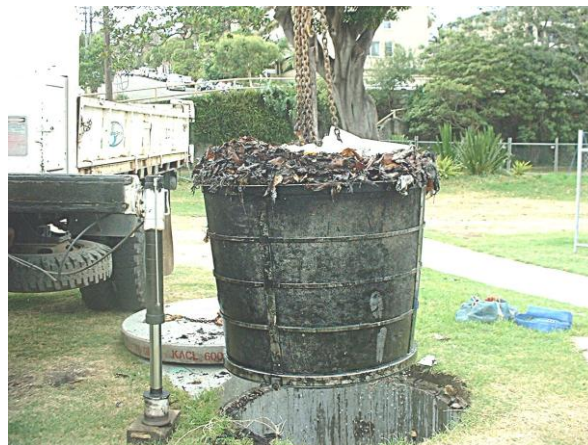
PLATE 6.1 EMPTYING THE BASKET CONTAINING THE SOLIDS IN A WET SUMP GPT
