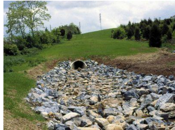
Photo 5 – Stormwater outlet protection
