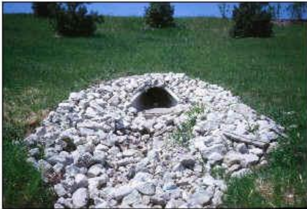
Photo 4 – Stormwater outlet protection
