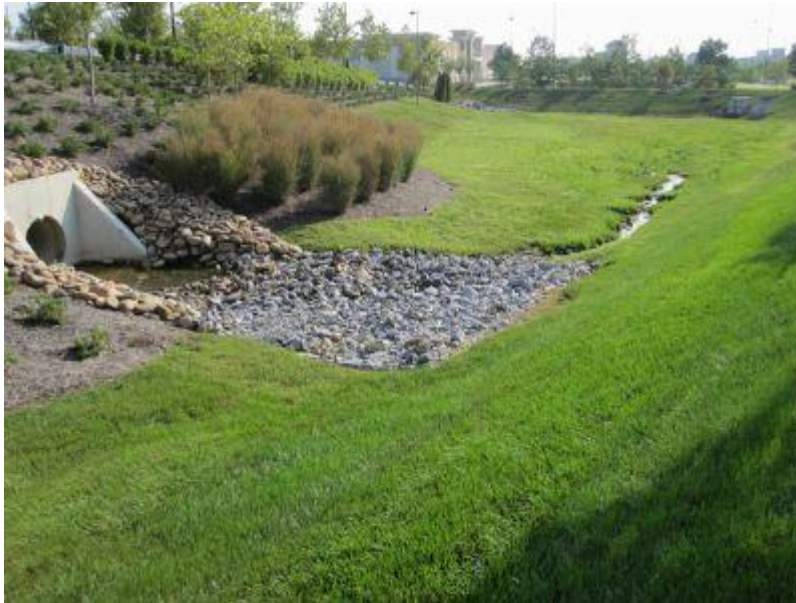
Photo 3 - Stormwater outlet protection
