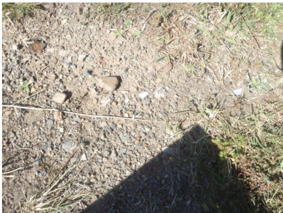
Photograph 9 Asbestos Cement debris adjacent to Test Pit 8
