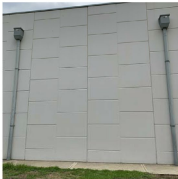
Existing pre-cast concrete panels to be retained. Existing downpipes to be retained.
