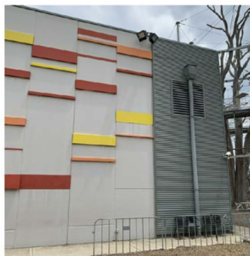
Existing pre-cast concrete panels with feature colour panels to be retained. Existing corrugated cladding to be retained.
