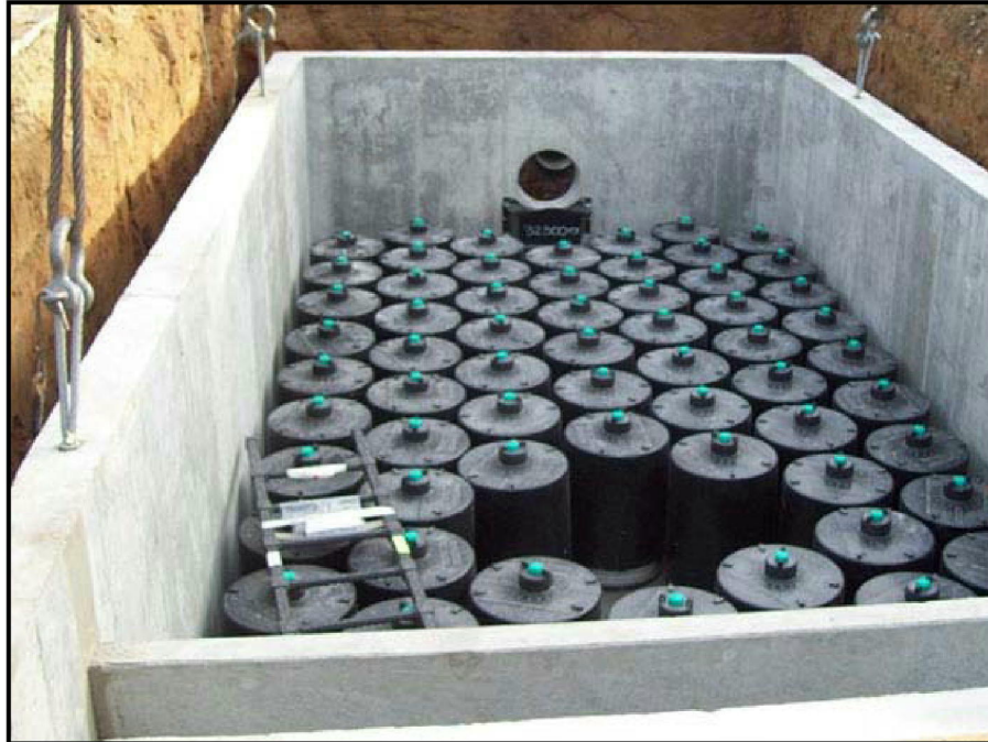
Plate 4.7 - Typical Cartridge Filter System (During Construction)
