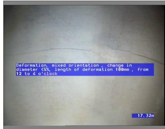
Photo: 35_1_3_08022014_130008_A.JPG 17.31m, Deformation, mixed orientation , change in diameter <5%, length of deformation 100mm , from 12 to 4 o'clock
