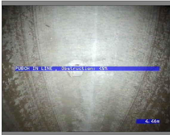
Photo: 23_1_2_08022014_111853_A.JPG 4.46m, PUBCH IN LINE , Obstruction: <5%
