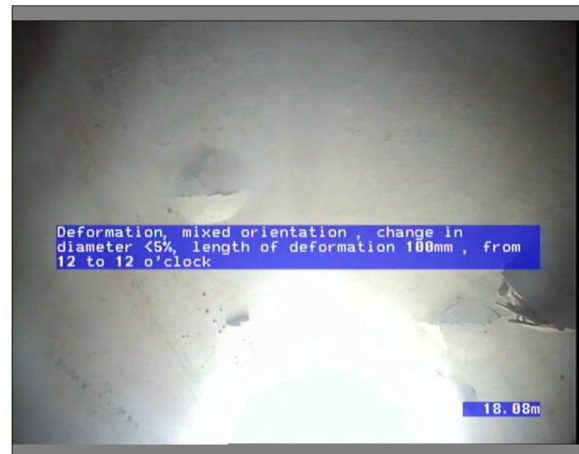
Photo: 35_1_5_08022014_130043_A.JPG 18.08m, Deformation, mixed orientation , change in diameter <5%, length of deformation 100mm , from 12 to 12 o'clock
