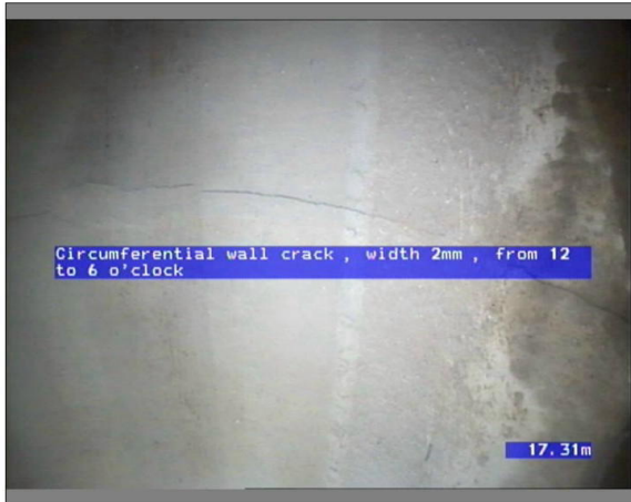
Photo: 35_1_2_08022014_125944_A.JPG 17.31m, Circumferential wall crack , width 2mm , from 12 to 6 o'clock
