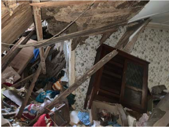
Figure 13: View of the collapsed first floor.
