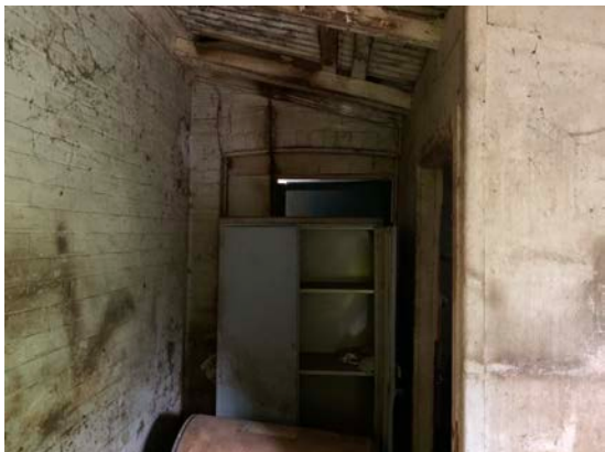
Figure 17: View of the semi-enclosed verandah on the western elevation, looking through to the remnant original brick vestry.
