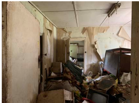
Figure 18: View of the kitchen in the skillion roofed additions on the eastern side of the building.
