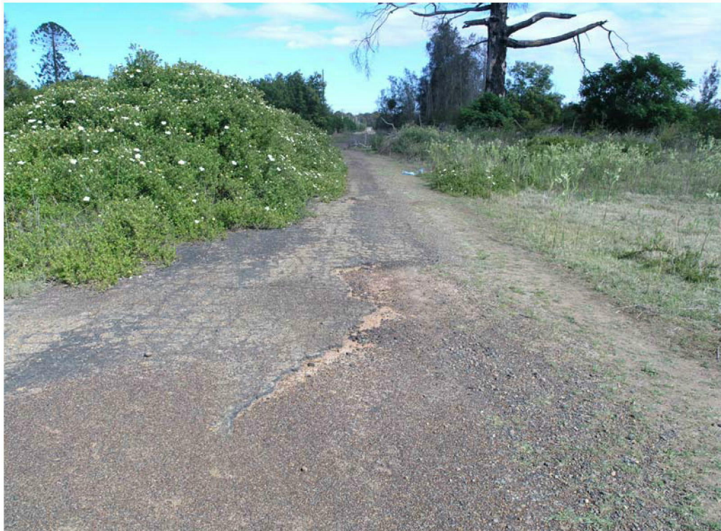
Plate 1: View along the former roadway leading to the Bridge showing made surface.
