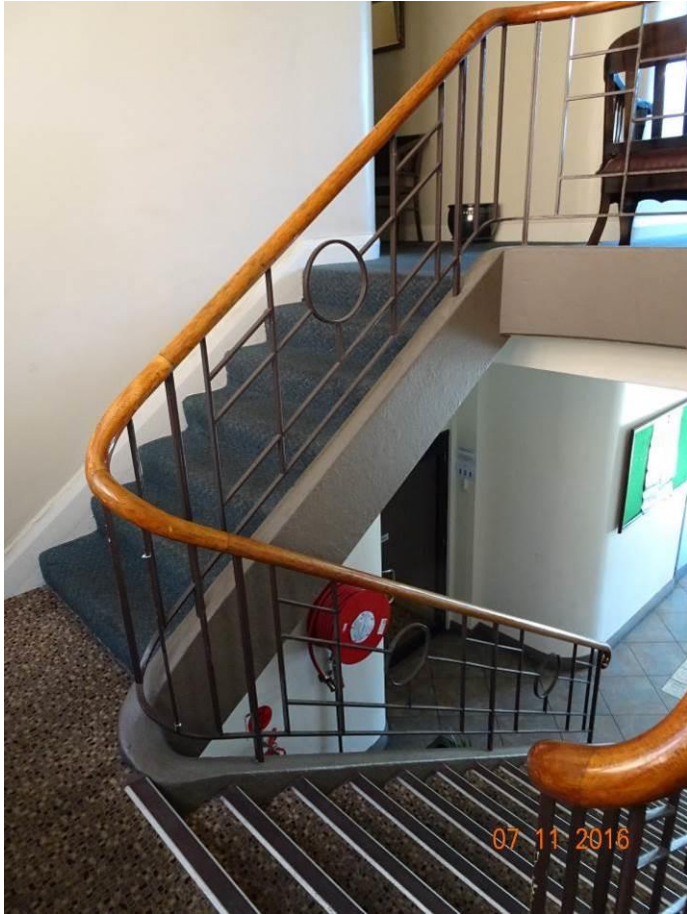
Figure 41: Stair balustrade and curved handrails
