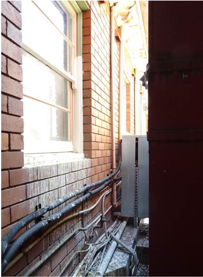
Figure 31: First Floor Eastern side showing services pipework
