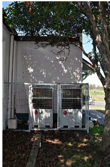
18. Condenser units- south wall.
