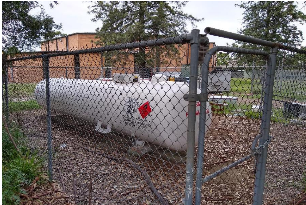
Photo 6 - LGP ASTs in central northern portion of site
