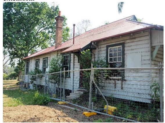
Figure 6: East elevation of the former Police Station and Residence, with original main entry.
