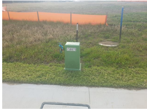
Underground electrical supply
