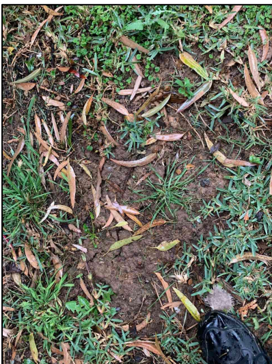
Figure 6: Showing heaving soil around the base of Tree 8.
