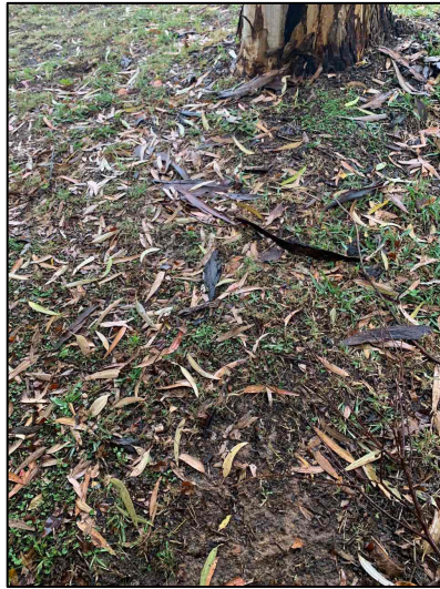
Figure 4: Showing heaving soil around the base of Tree 8.
