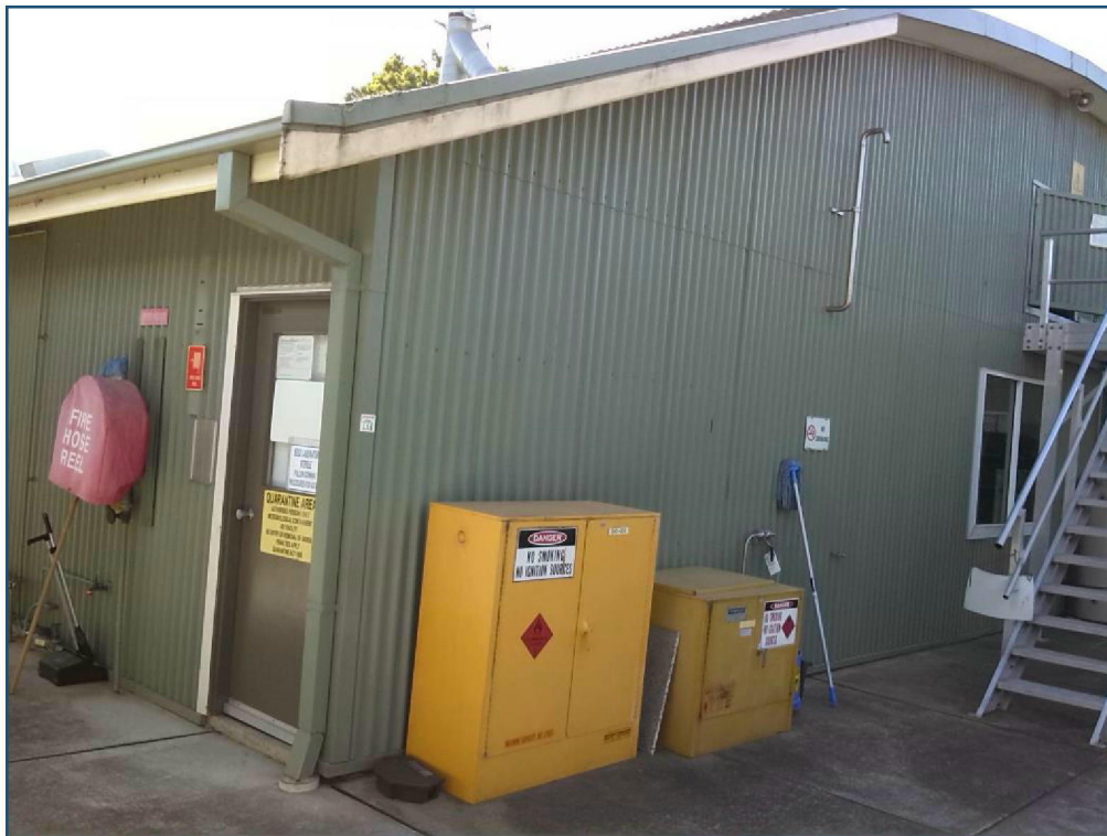
b) Existing single storey enclosure which is to be increased in area with 2.8 m x 2.0 m addition. New works to match existing building as closely as possible.
