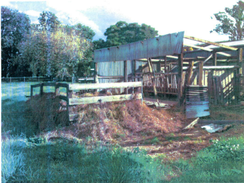
Figure 5 - Rear of former calf feeding shed showing timber framed extension to enclosed area and adjoining feed box.
