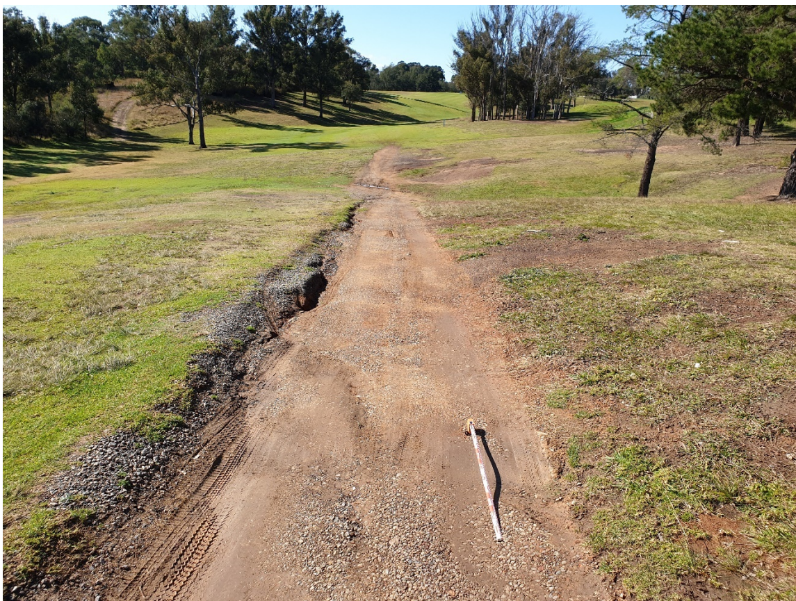
Figure 5.6 East facing view showing repeated erosion on path and within gully (1m scale).
