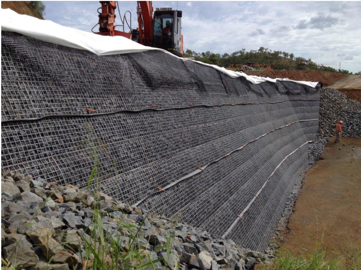
Plate 1 Typical stone filled steel mesh structure to face of wall (Photo supplied: Enviroguard Pty Ltd)
