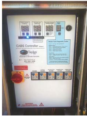
CABS Control Panel
