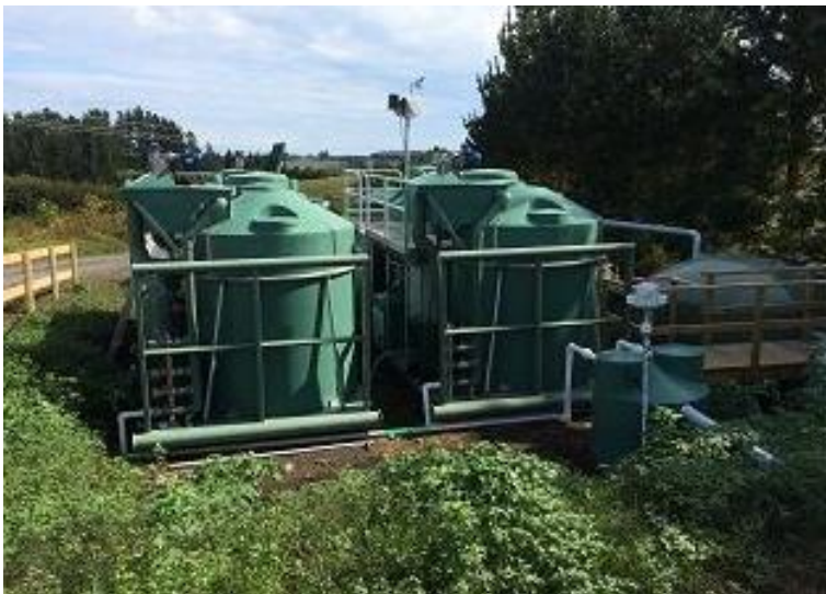
Figure 11 Site equivalent: balance/settlement, two SK20 SBR units, treated effluent tank and pump
