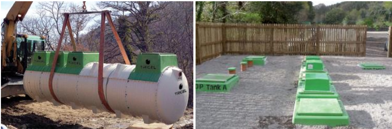
Figure 12 Site equivalent: balance/settlement, two Tricell units, treated effluent tank and pump
