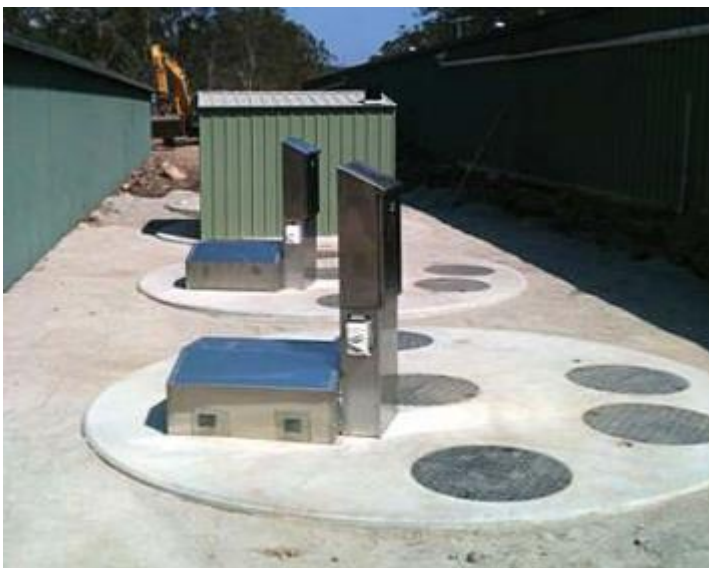
Figure 14 Ecowise system discretely installed below ground
