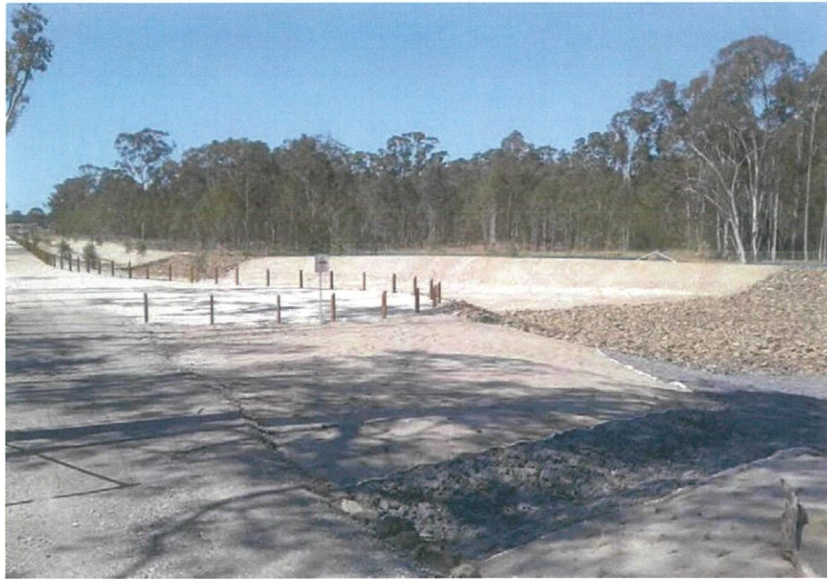
Photograph 5 - Engineered drainage system located to the south of the site
