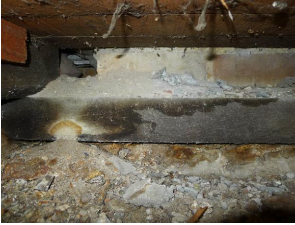
Figure 12: Evidence of fungal growth to bearers of Living Room Gallery subfloor.
