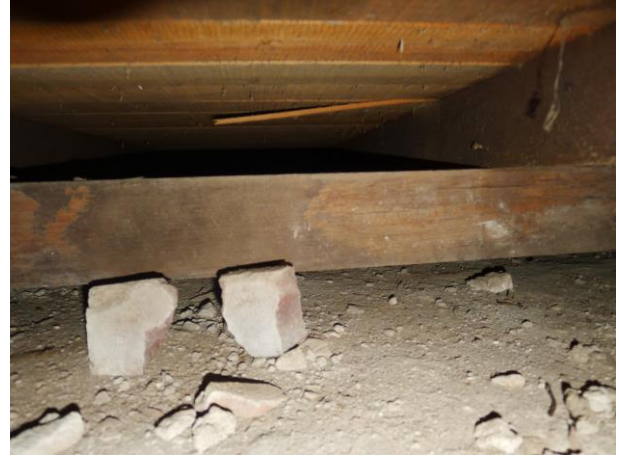
Figure 13: View of floor substructure of Living Room Gallery. Bearers are largely propped by bricks.
