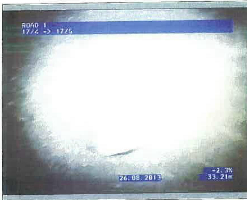
Photo: 33_1_2_02092013_162657_A.jpg 33.21m, Horizontal deformation , change in diameter 5-10%, length of deformation 100mm , at 3 o'clock
