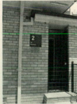
Photograph: View of existing entrance from East elevation – access from Piazza, with non-complaint entry.
