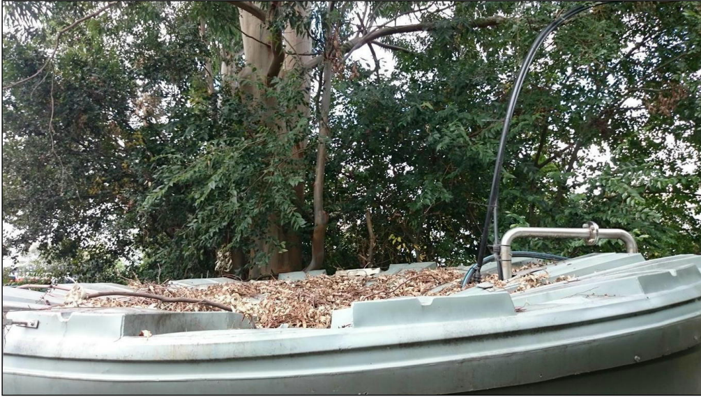
e) Damaged roof of existing tank proposed to be removed.
