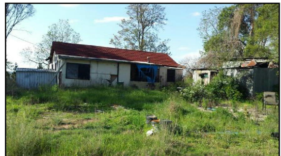
Dilapidated former dwelling and Outbuildings, to be demolished
