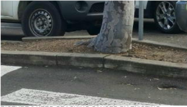
PICTURE 3 KERB CRACKING CAUSED BY EXISTING TREES
