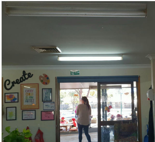
Fig – Lighting and Emergency lighting
