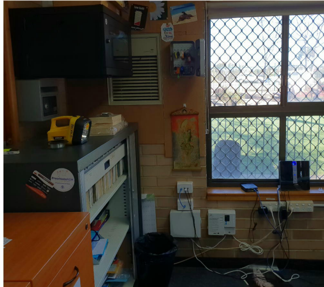
Fig –NBN equipment and power/data outlets
