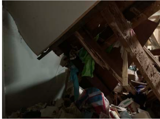
Figure 14: View of the collapsed first floor.
