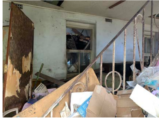
Figure 20: View of the ground floor on the northern elevation, showing the internal stair access to the first floor and masonry wall of the original church building.
