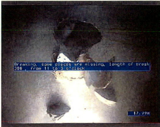
Photo: 35_1_4_08022014_130025_A.JPG 17.99m, Breaking, some pieces are missing, length of break 300 , from 11 to 3 o'clock
