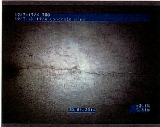
Photo: 193-194_193_194_30012014_080604_A.JPG 5.11m, Circumferential surface crack , width 1mm , from 8 to 4 o'clock
