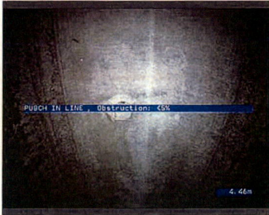
Photo: 23_1_2_08022014_111853_A.JPG 4.46m, PUBCH IN LINE , Obstruction: <5%
