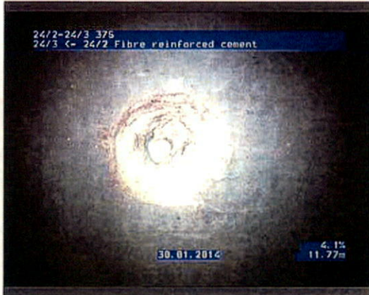
Photo: 242-243_242_243_30012014_123306_A.JPG 11.77m, Point repair, hole repaired, length: 50mm, repaired externally, at 1 o'clock
