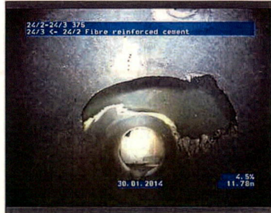
Photo: 242-243_242_243_30012014_123406_A.JPG 11.94m, Point repair, hole repaired, length: 1000mm, repaired externally, from 10 to 3 o'clock
