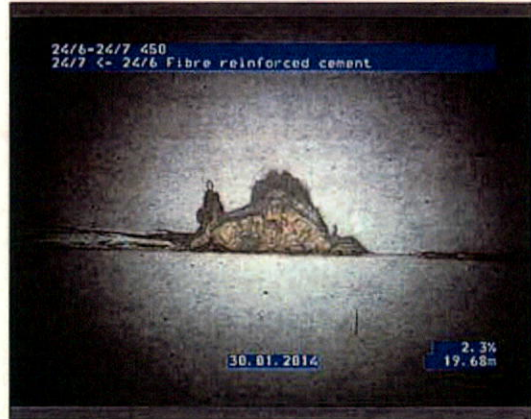
Photo: 246-247_246_247_30012014_142036_A.JPG 19.68m, Breaking, some pieces are missing, length of break 100, at joint, at 12 o'clock
