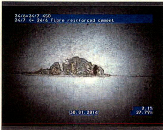
Photo: 246-247_246_247_30012014_142208_A.JPG 27.79m, Breaking, some pieces are missing, length of break 100, at joint, at 12 o'clock
