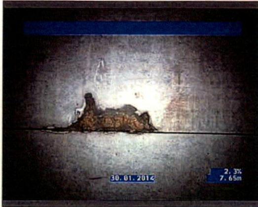
Photo: 246-247_246_247_30012014_141914_A.JPG 7.65m, Breaking, some pieces are missing, length of break 100, at joint, at 12 o'clock
