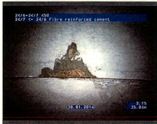
Photo: 246-247_246_247_30012014_142312_A.JPG 35.84m, Breaking, some pieces are missing, length of break 100, at joint, at 12 o'clock
