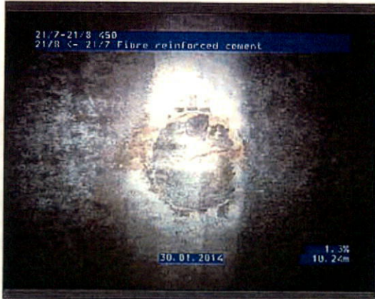
Photo: 217-218_217_218_30012014_092123_A.JPG 10.24m, Breaking, all pieces are present but some of them are visibly displaced from position, length of break 100 , at 7 o'clock
