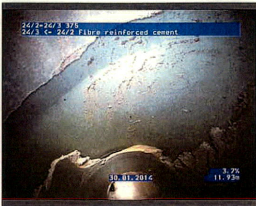
Photo: 242-243_242_243_30012014_123413_B.JPG 11.94m, Point repair, hole repaired, length: 1000mm, repaired externally, from 10 to 3 o'clock
