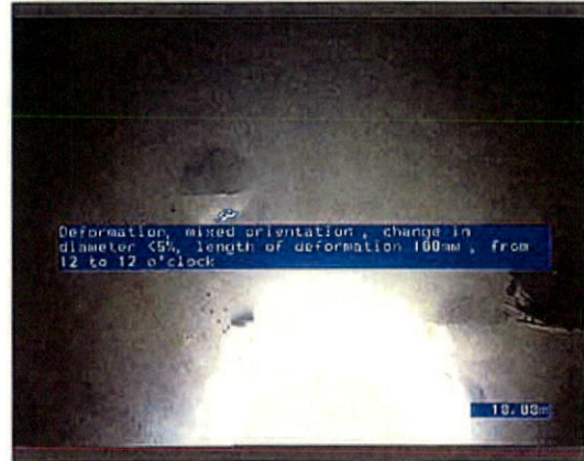
Photo: 35_1_5_08022014_130043_A.JPG 18.08m, Deformation, mixed orientation , change in diameter <5%, length of deformation 100mm , from 12 to 12 o'clock
