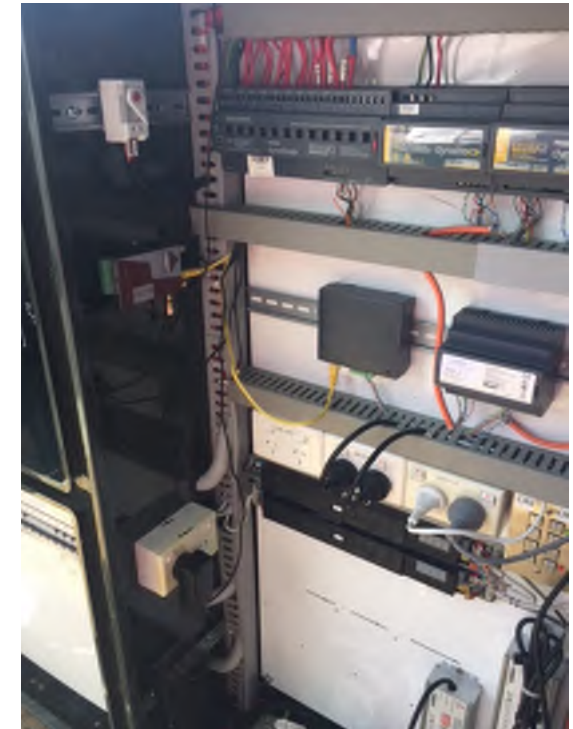
Lighting Control Equipment
