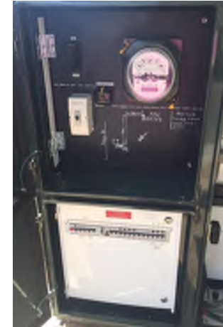
Distribution Board and Metering
