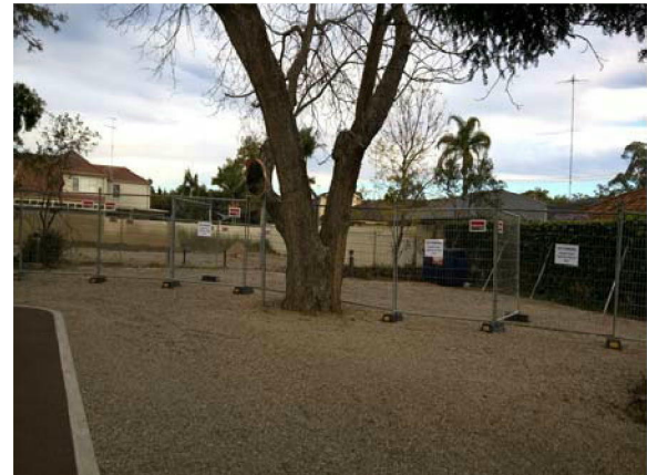
Photograph Southern west corner of boundary Southern section of collapsed wall removed, western section supported – vegetation covering wall.
