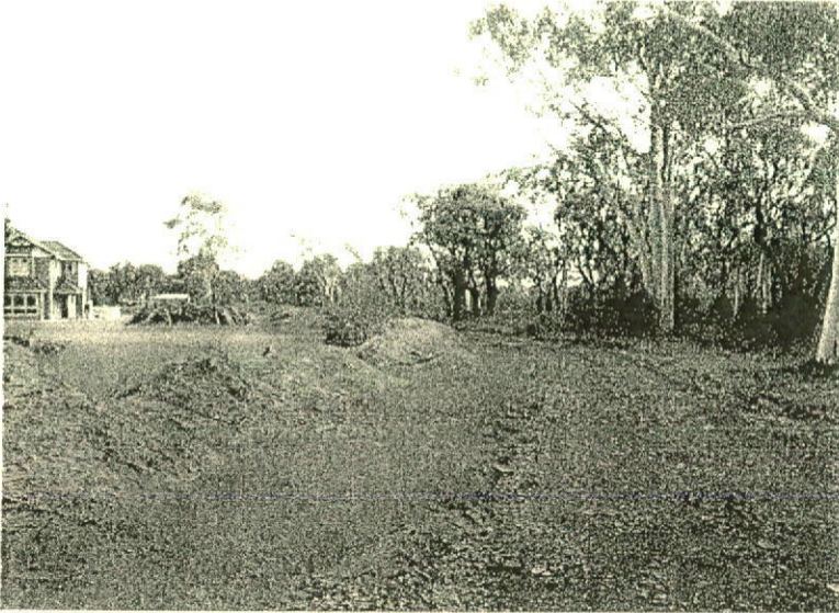
Natural excavated material from the site to be used for top soiling of property
