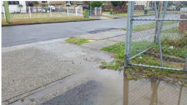
Photo 4: Carpark discharges over footpath to kerb
