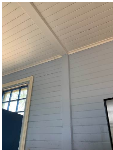
Figure 3. 80: S9 (kitchen) with evidence of location of former partition in ceiling and west wall.
