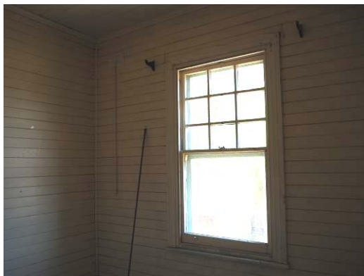
Figure 3. 68: Window in S5 (bedroom).
