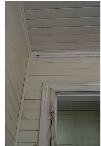
Figure 3. 90: Evidence of location of former light pull in cornice in Space S5
