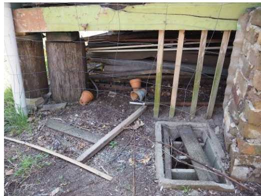
Figure 3. 54: View of roof sheeting and other building elements stored under the building.
