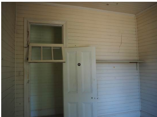
Figure 3. 67: S5 (bedroom) with door and broken fanlight.
