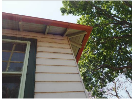
Figure 3. 52: Detail of external weatherboards and timber panelled soffits and exposed eaves rafters.
