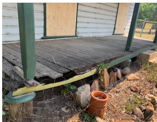
Figure 3. 50: Condition of timber flooring to north (front) verandah
