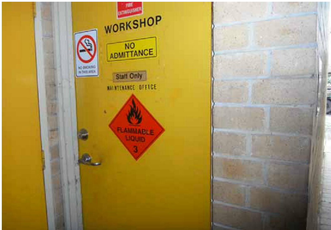
Photo 9 - Door to workshop indicates storage of flammable liquids
