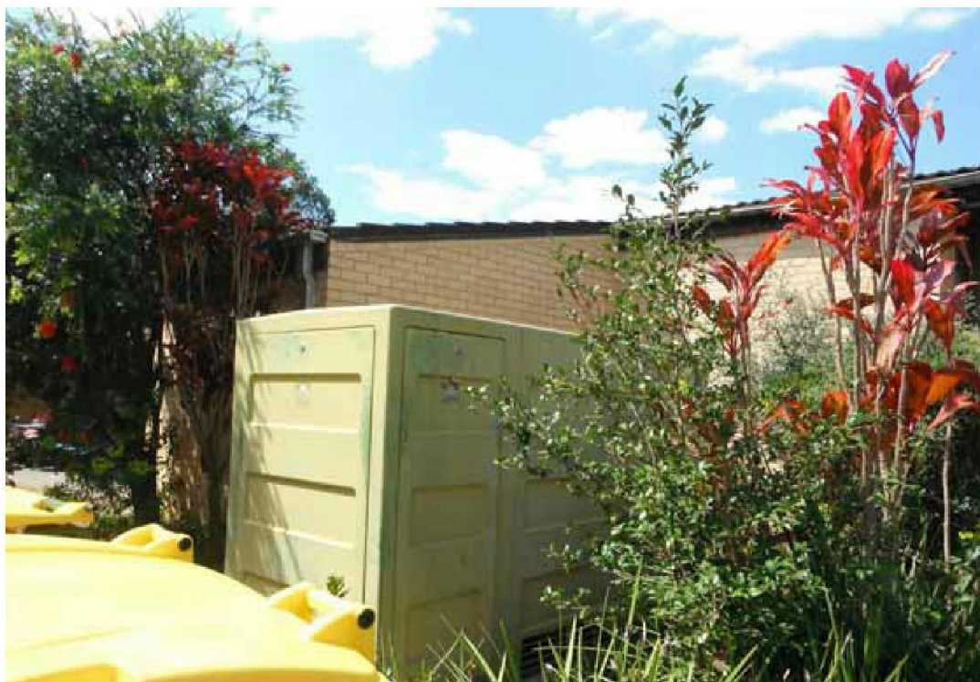
Photo 4 - Substation observed adjacent Emerald Street access driveway
