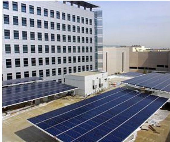
Figure 13 PV on roof structure
