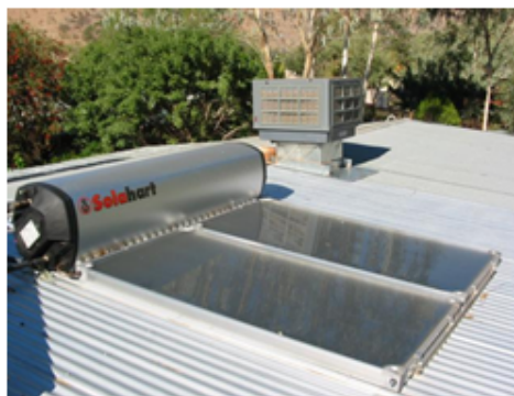
Figure 14 Solar hot water system
