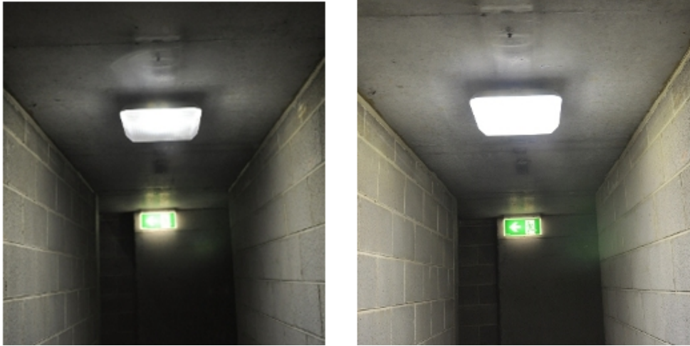
Figure 11 Emergency lights in standby & occupancy modes
