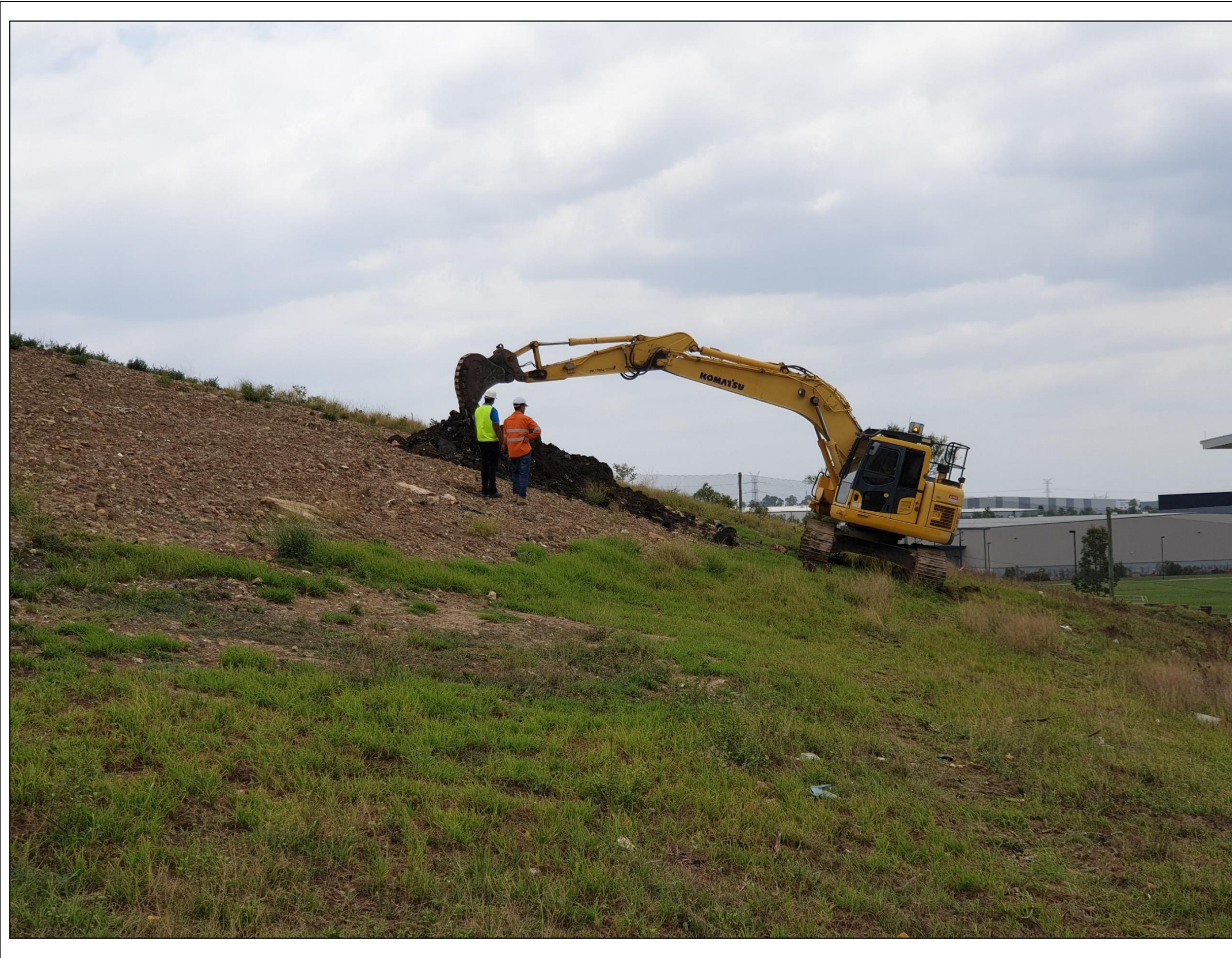
Photo 3.3 – Excavation of bore hole test location (Pit 2) sampled by TOU on 4 February 2020
